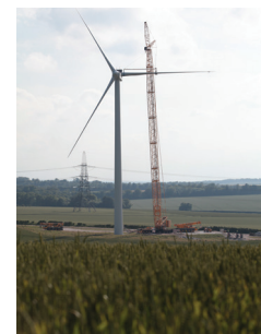
4. Once final checks are completed, the turbine is ready to generate renewable energy
